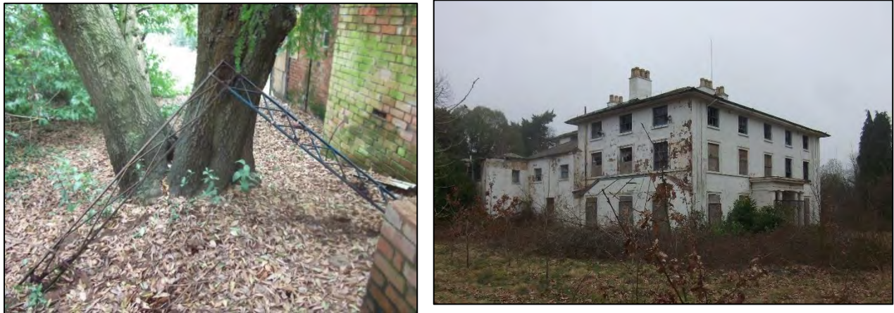
Figure 23: Detail of the Loggia structure (left) and the west and south elevation of the main house showing the roof line (right). Unlike the East elevation, the western elevation comprises a three storey section of 3 windows with an adjacent 2 storey structure
