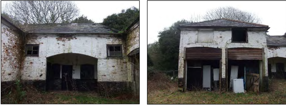
Figure 30: The central section of the Coach House looking towards the east in 2021
