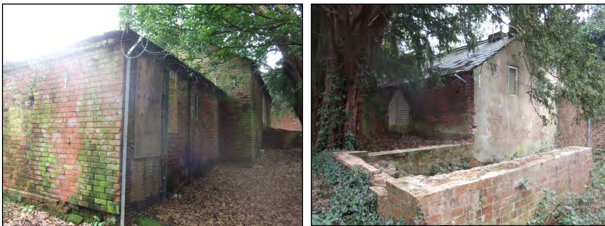
Figure 27: (left) Corner of the East Wing, showing the adjoining single storey structure (right) which forms the northern boundary to the inner courtyard.
