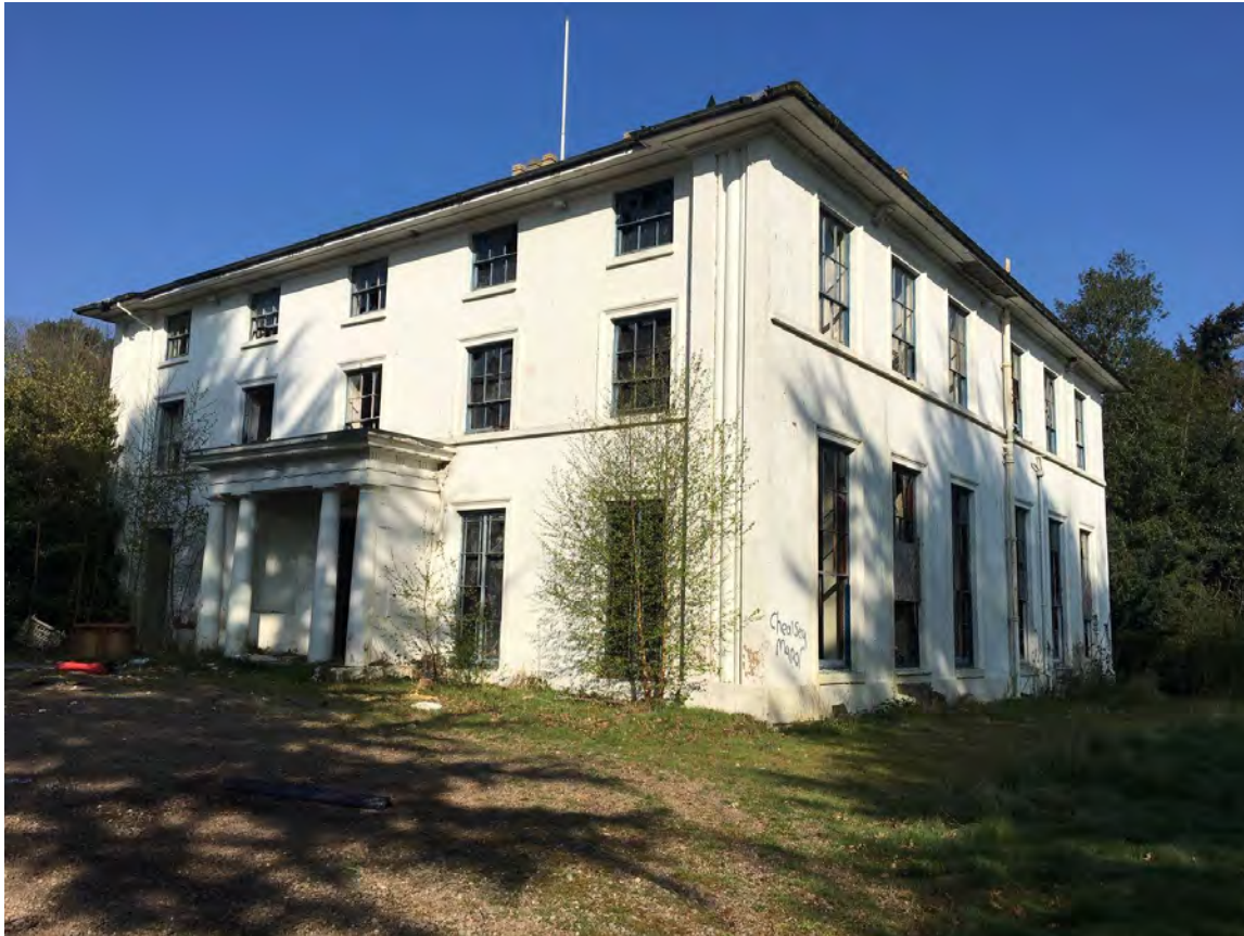
Figure 22: The front and east elevation of the main house prior to boarding up showing casement windows to ground floor of the south elevation and 9/6 sashes to the east elevation
