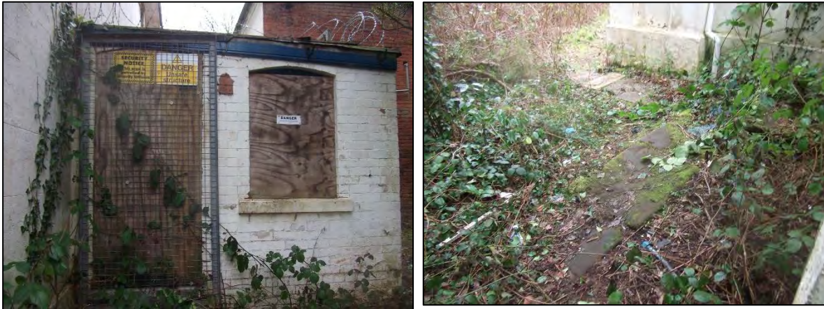
Figure 26: (left) Later addition, possibly serving the garden with (right) evidence of flags or footings in front of it
