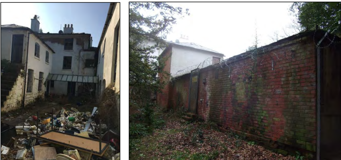
Figure 25: Left: The rear courtyard looking towards the main house. The East Wing is to the left and shows the two storey laundry/kitchen. Right: The east elevation of the East Wing with blocked doorway
